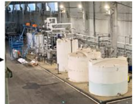
REE Recovery Pilot Plant (Jan 2021)
